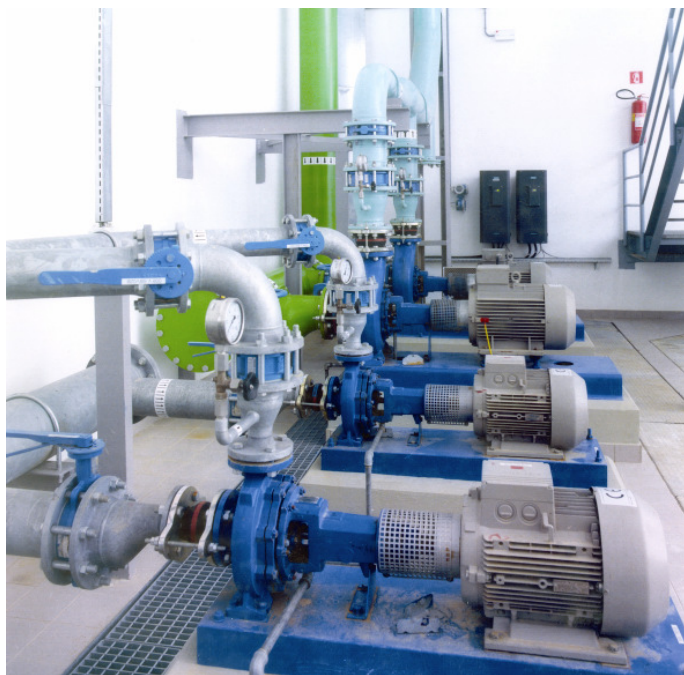
Water and Sewage Treatment Plants are Ideal Candidates for Fieldbus Technology Due to the Harsh Operating Environments and the Long Distances Between Controllers and Devices
